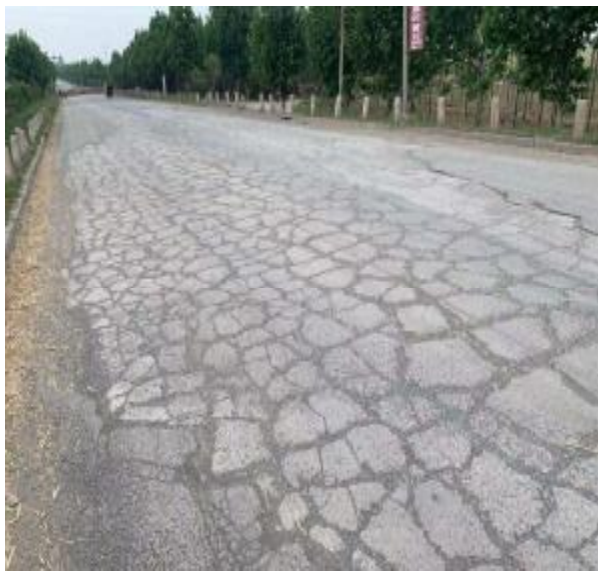
顺接桥梁路面网裂
